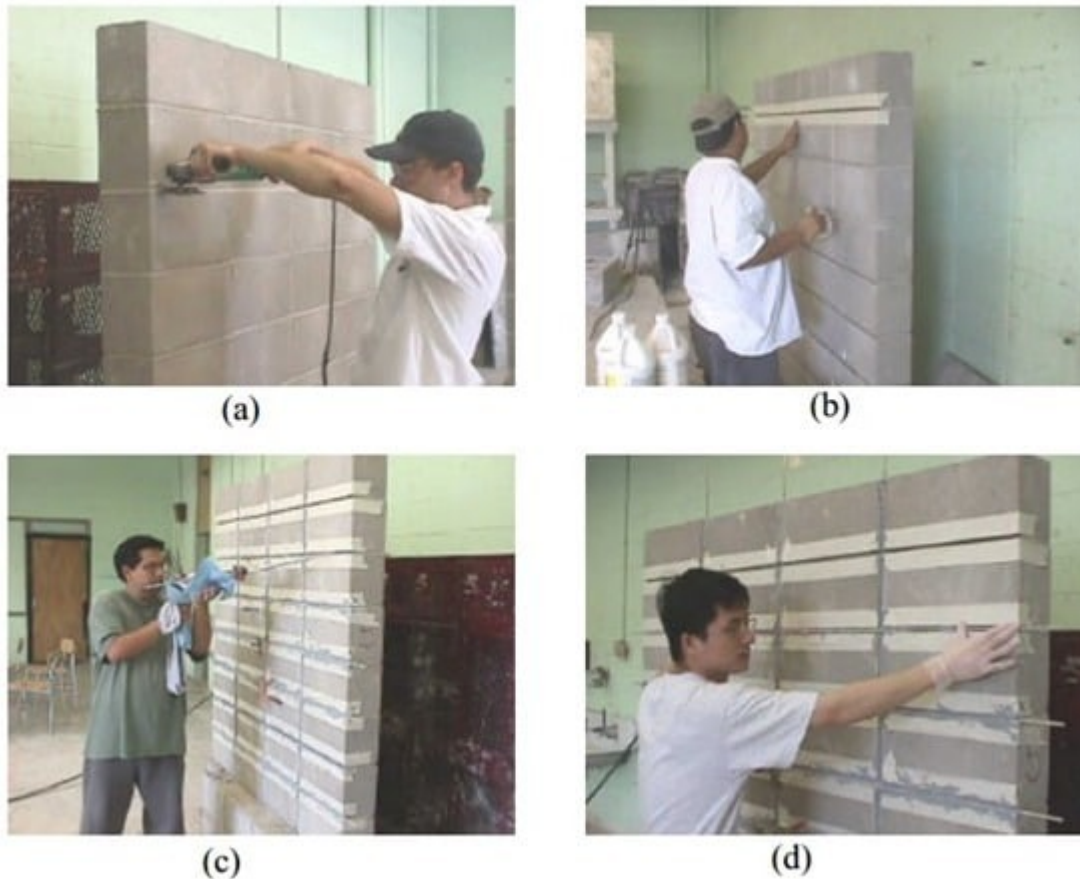
Fig: Strengthening of Masonry Walls using FRP Structural Repointing; (a) Grinding of masonry joints, (b) Masking of masonry to avoid staining, (c) Application of epoxy based paste to masonry joint, (d) Installation of GFRP Rod
